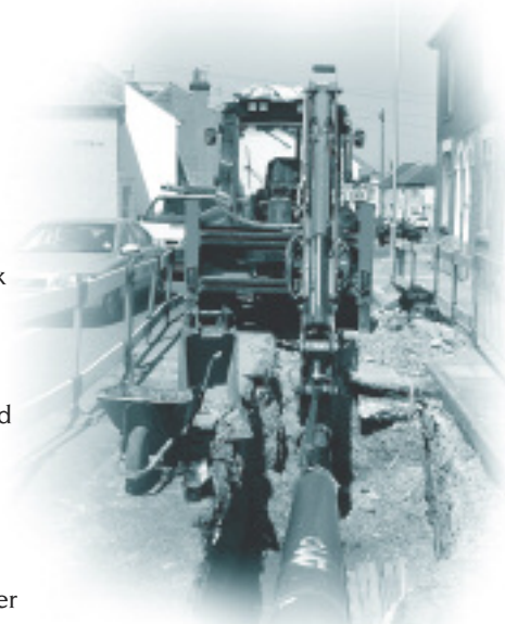
Inserting a new main inside the old one in Eastney Road, Portsmouth
