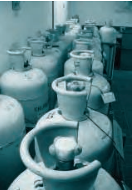
Chemical storage at a treatment works
