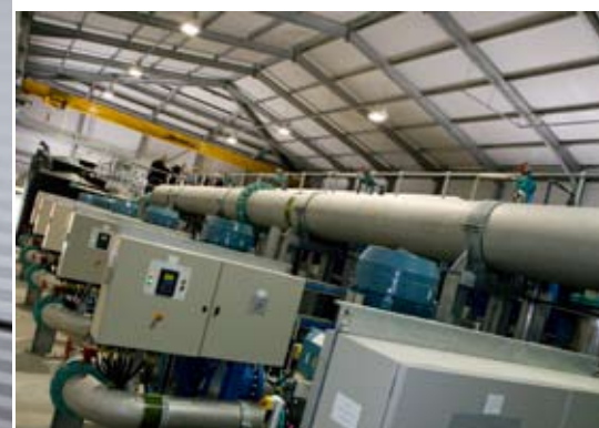
BELOW The River Itchen Works Membrane Filtration Plant
