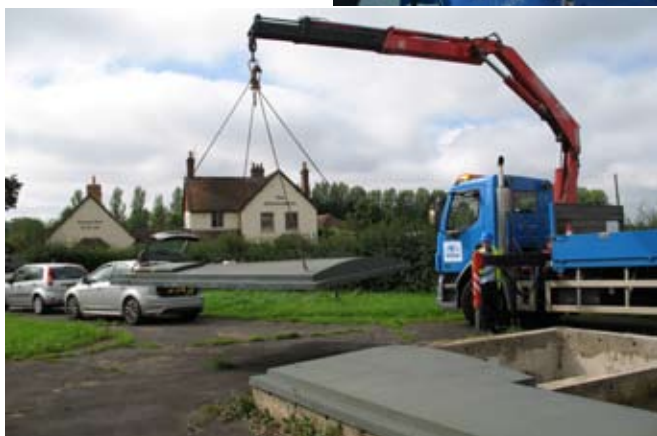
BELOW Replacing a borehole headworks cover at World's End Water Treatment Works
