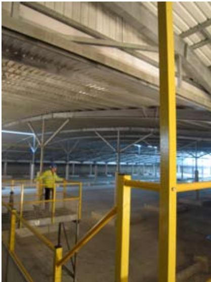
View from the inside of the large compartment of Highwood raw water reservoir during capital scheme undertaken to construct a roof over the reservoir
