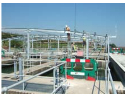
Steelwork installation connected with a capital scheme to cover rapid gravity filters at one of the Company's treatment works.
