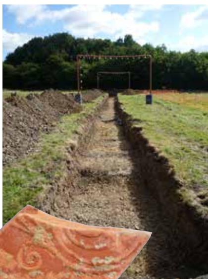
Trench dug for mains renewal scheme at Fishbourne Roman Palace. A number of artefacts were found on the site, including the item shown left.
